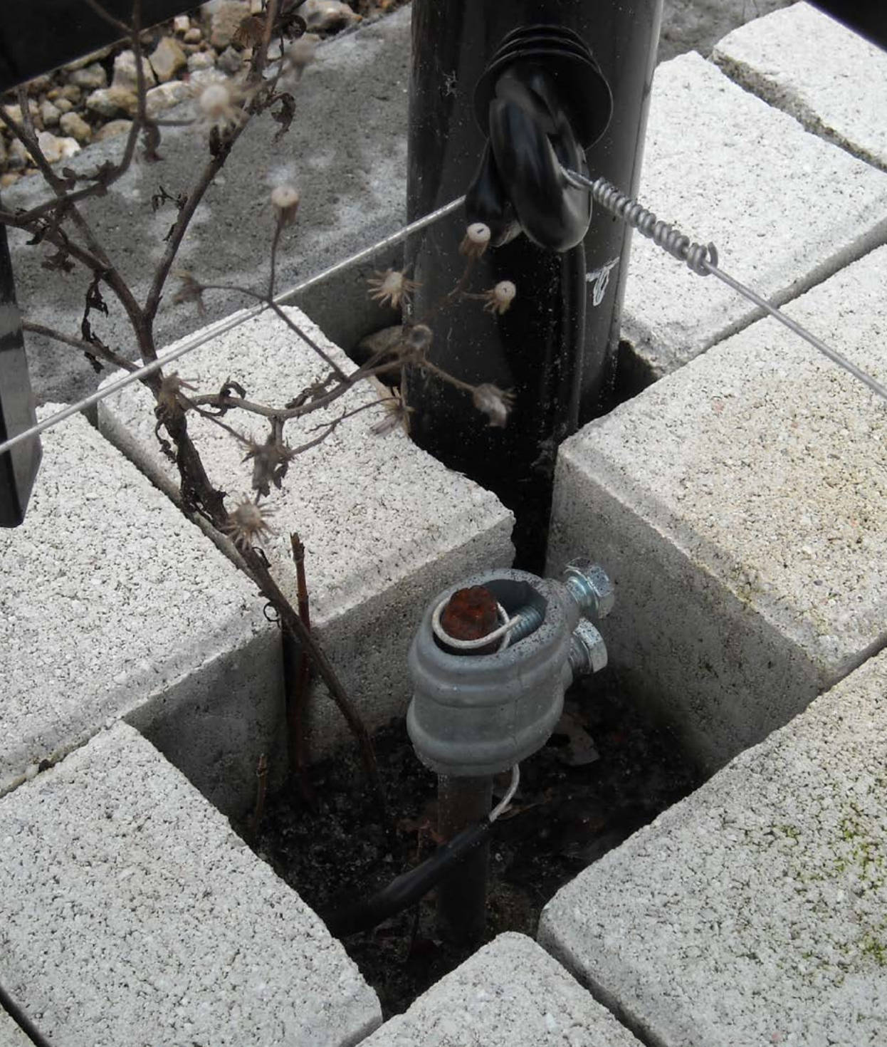
Ground rods like these can be used to divert the peak voltage of a lightning strike to the ground. This is very important, and especially if the project includes electric gates.
